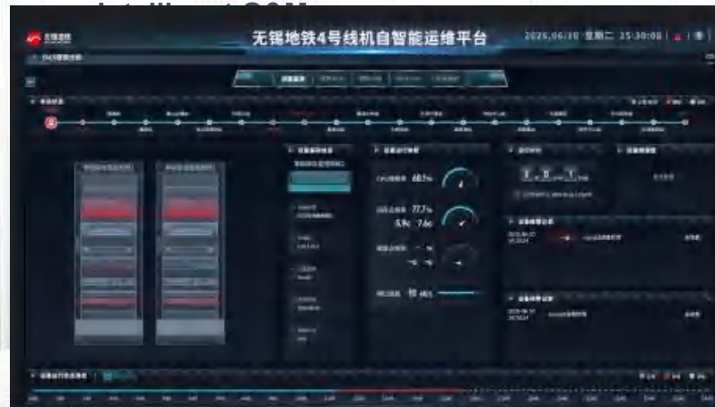
Integrated Supervisory Control Host Performance Monitoring
